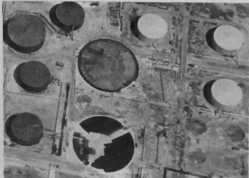
FOUNDATIONS OF two new 400,000 bbls. tanks now under construction in Tank Farm.
